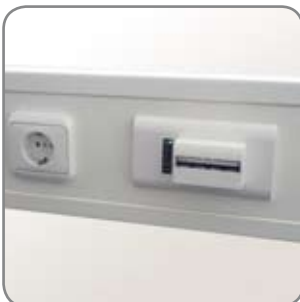
Installation in cable duct
